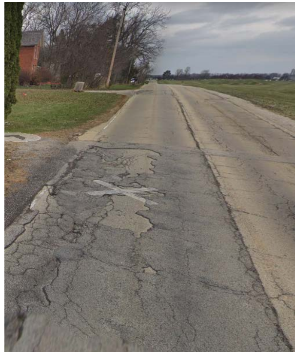
Figure 10: Kautz Road condition
